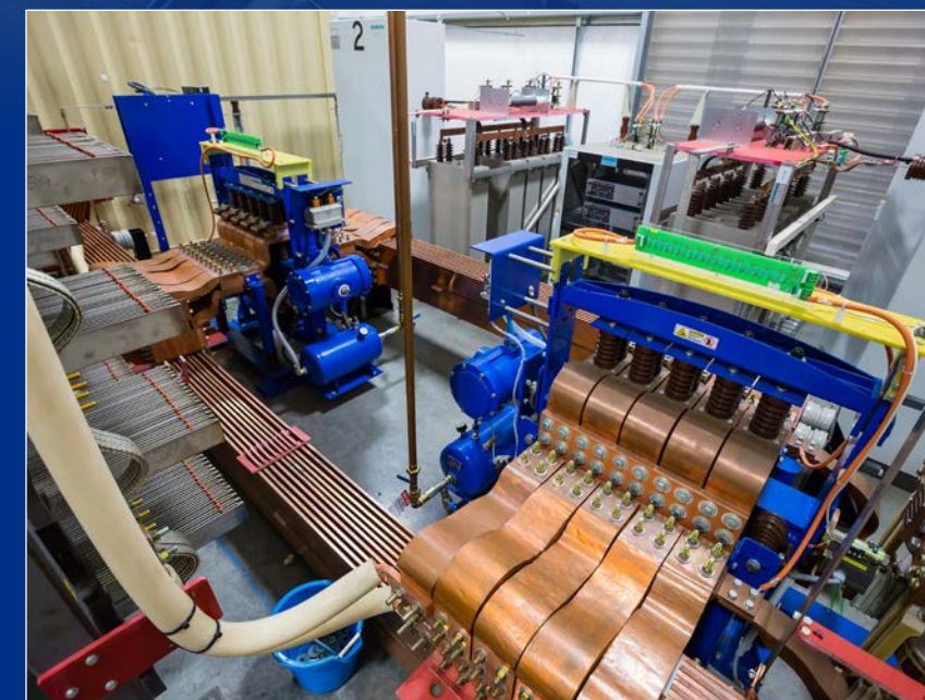
50kA magnet charging power supply with 1GJ fast discharge system including 7kV DC switch and dump resistor for full-current testing of CS modules
