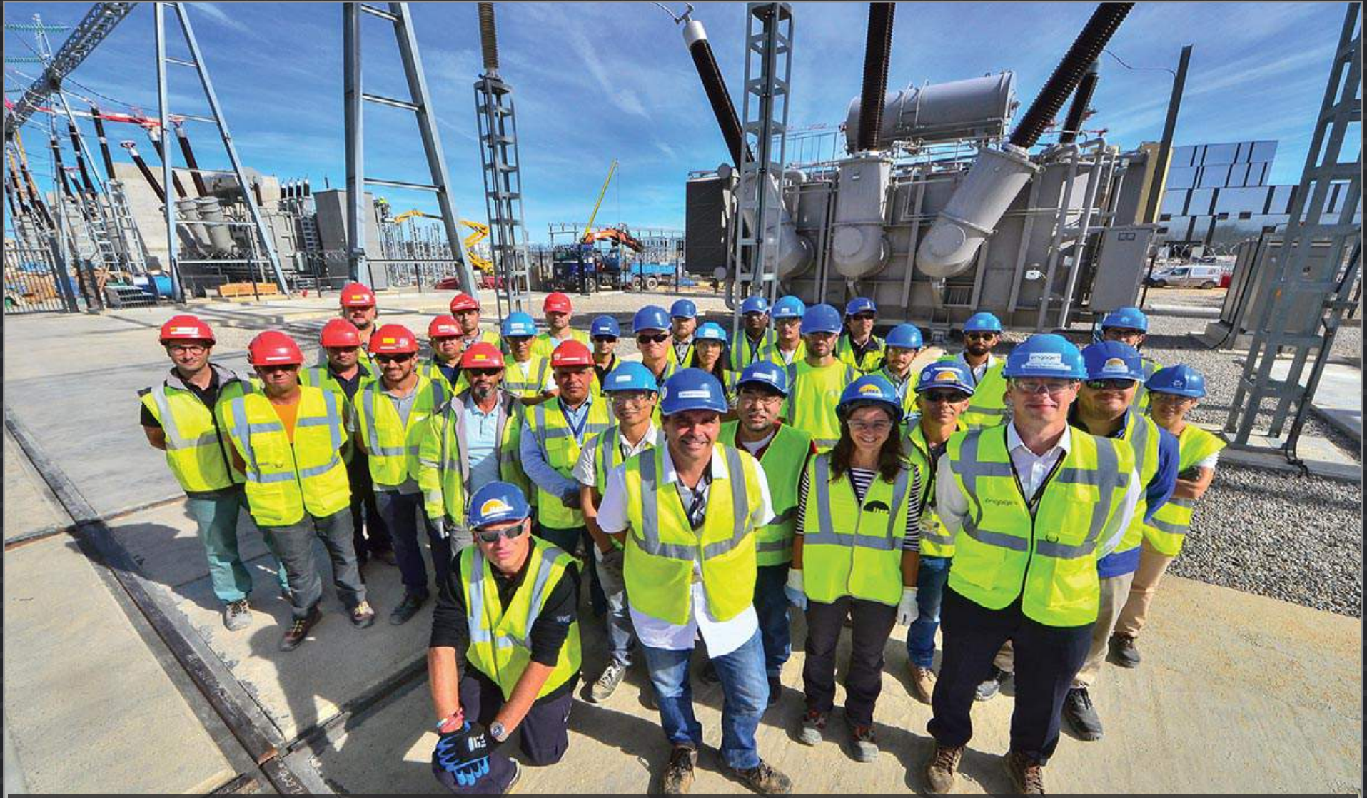
Four transformers supplied by US ITER for the steady state electrical network have been "energized" and ITER is officially connected to the French grid. September 2018
