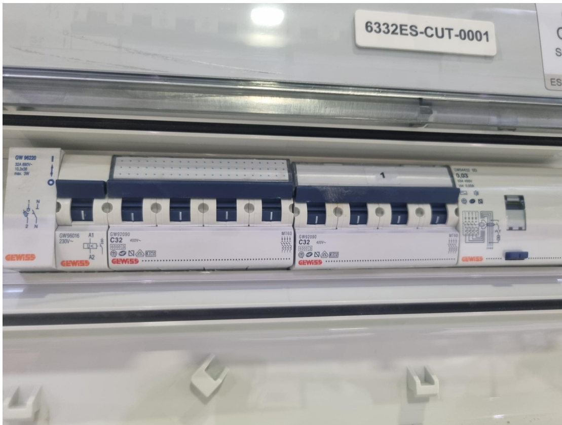
Figure 18 Zoom of the protections in the power supply 32 A – 16 A
