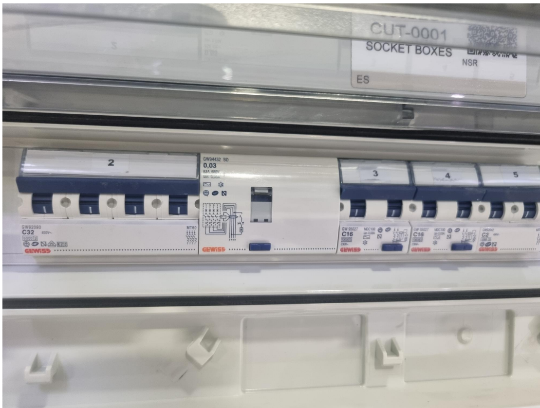
Figure 19 Zoom of the protections in the power supply 32 A – 16 A
