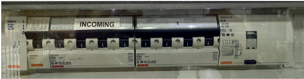
Figure 20 Zoom of the protections in the power supply 63 A - 16 A
