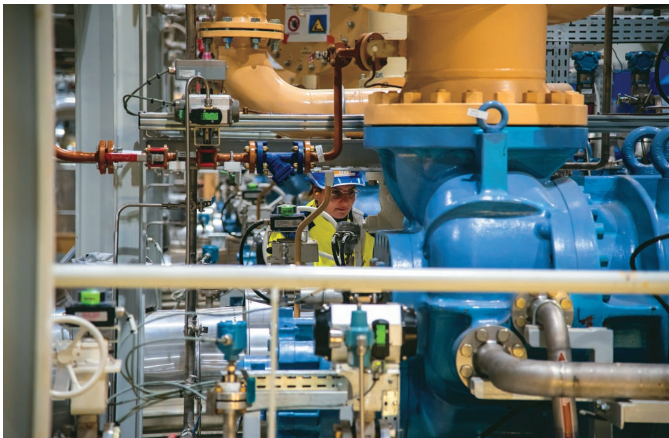
▲ Helium was compressed for the first time in the cryoplant this year as part of commissioning activities.
