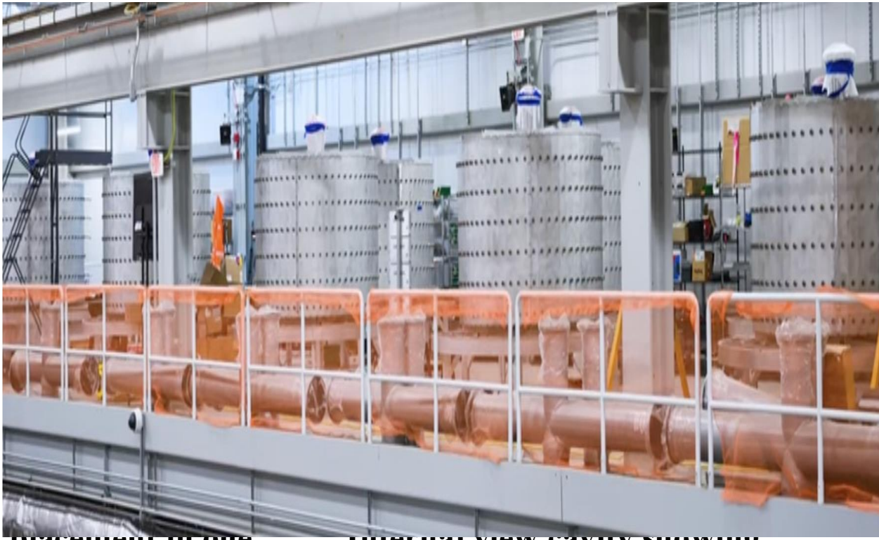
Internal view cavity showing coupling loops and transmission line
