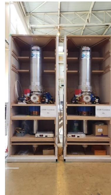
JADA gyrotrons at ITER site
