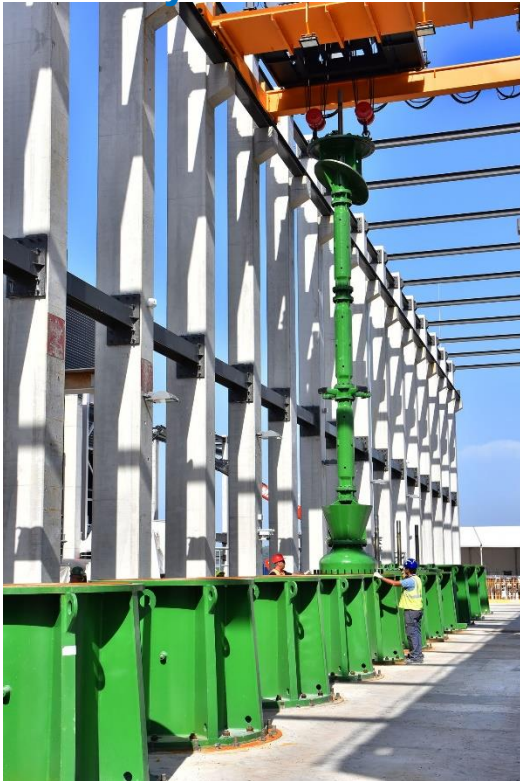
Vertical Pumps for HRS in assembly
