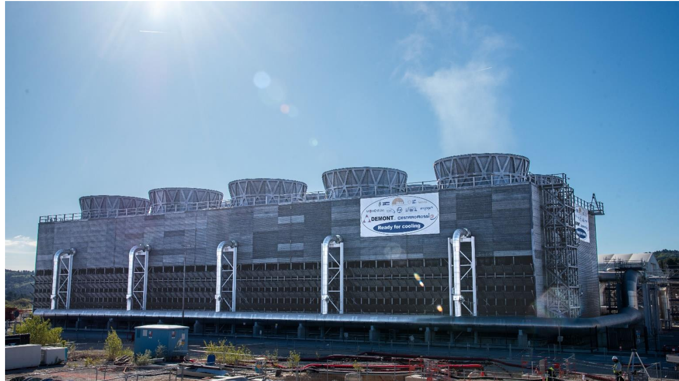
Heat rejection system in operation
