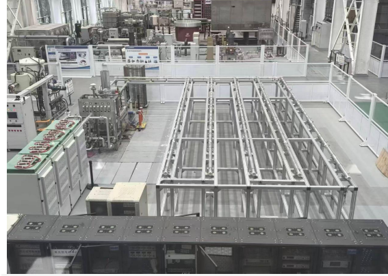
High-Power Long-Pulse 100-Meter-Class Transmission Line System Test Platform
