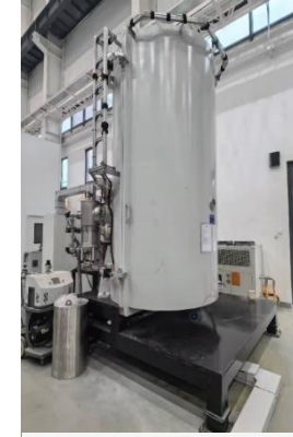
UHV Exhaust Station
