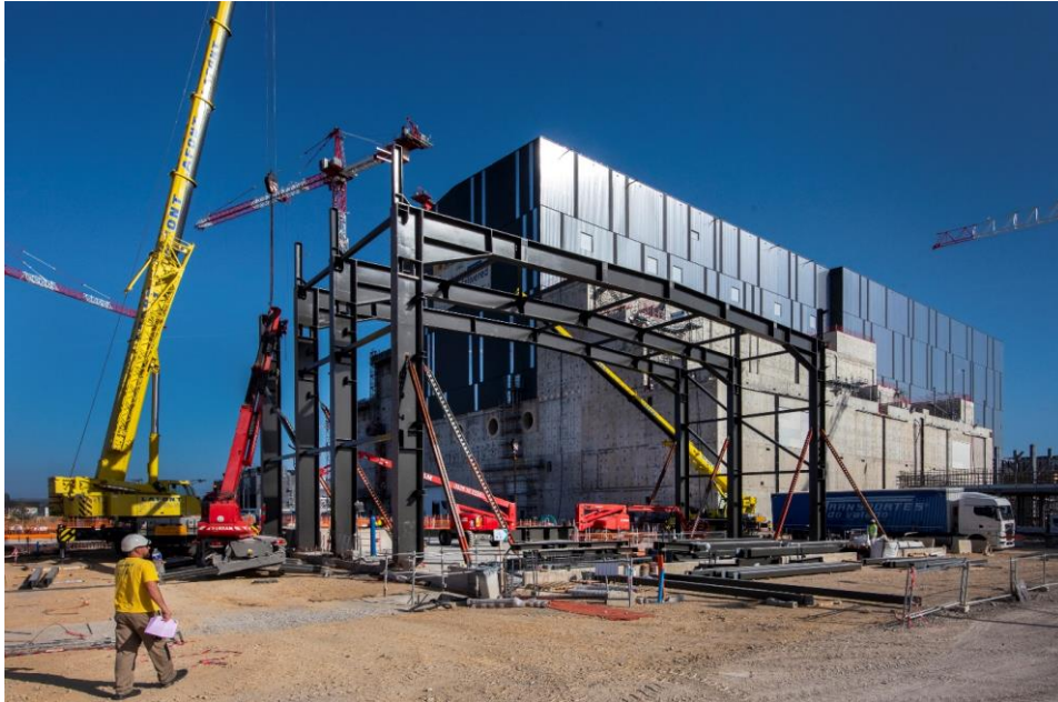
Fig. 8.4-45: metal structure of the neutral beam power supply's High Voltage Building.
